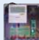
PCB, Power trans, Terminal block
